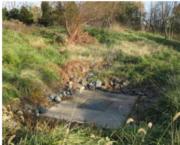
Concrete Stormwater Collection
