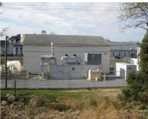
Landfill Gas-to-Energy Facility
