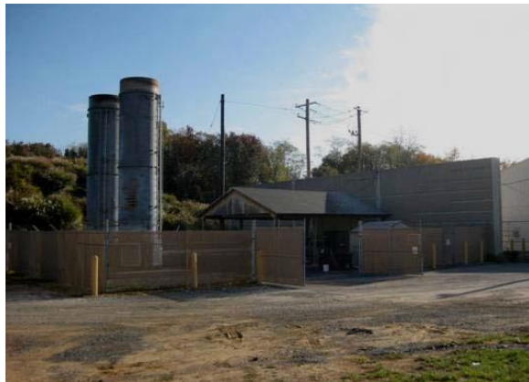
Landfill Gas Flare Station
