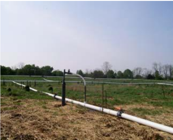
Landfill Gas Extraction Well & Piping
